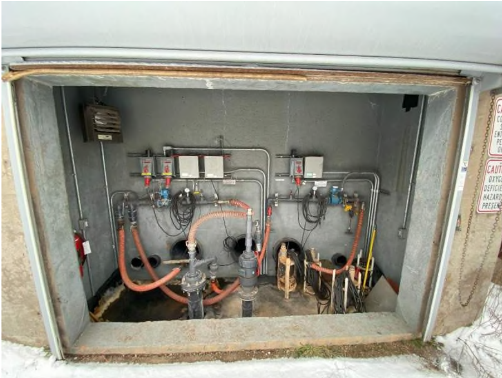
Photo No. 1 – Landfill No. 3, Cell 2 leachate collection riser vault.
