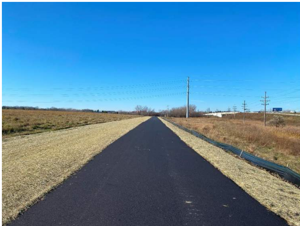
Photo No. 4 – North slope of Cell 1, looking west. Asphalt perimeter road was installed in 2024.
