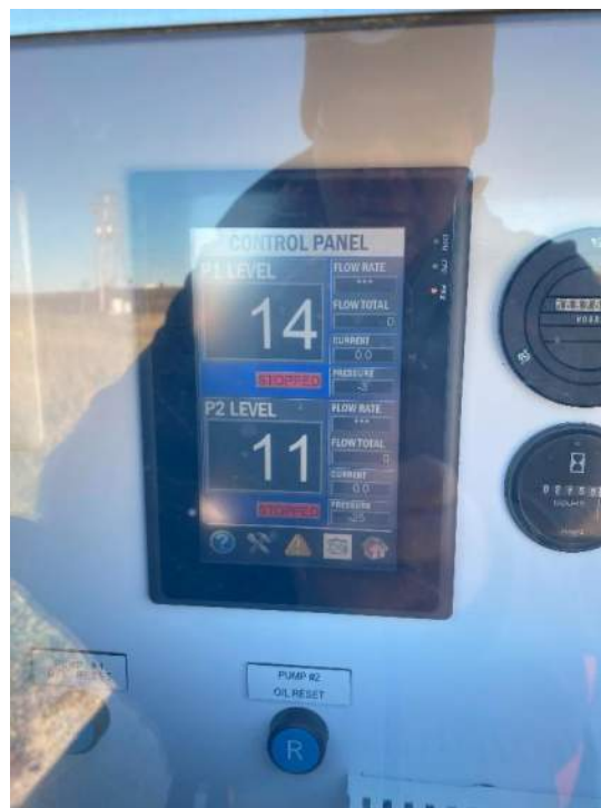
Photo No. 10 – Leachate loadout screen.
