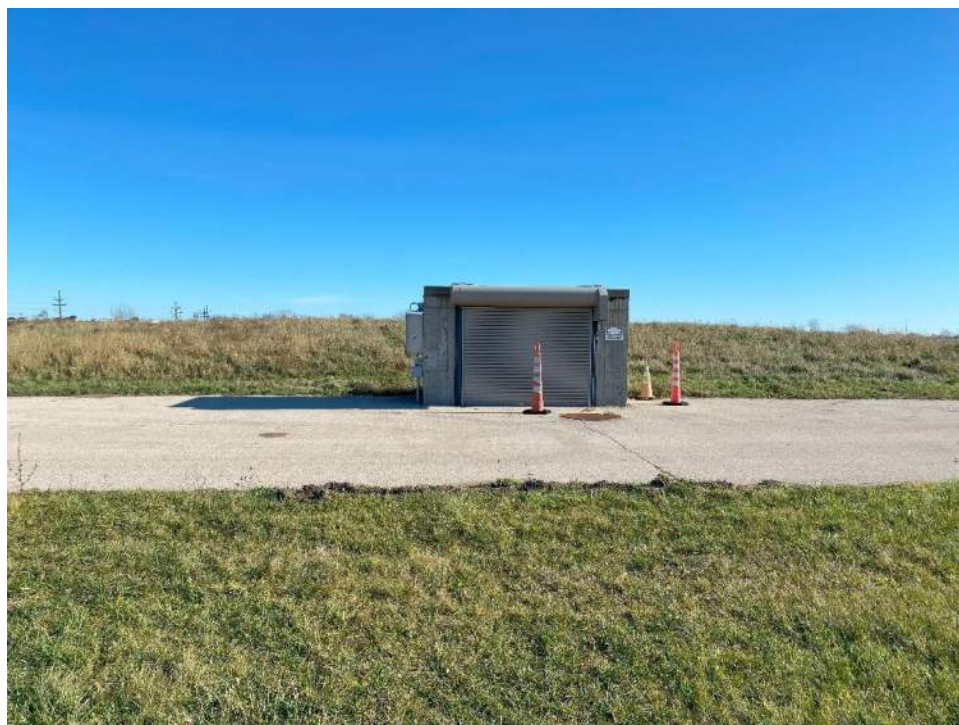
Photo No. 2 – Leachate sump collection vault.
