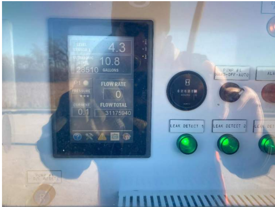
Photo No. 1 – Leachate loadout screen.
