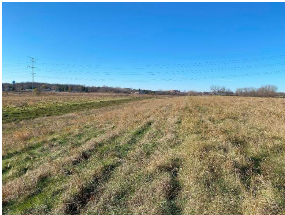
Photo No. 6 – South slope of Cell 1 and perimeter stormwater ditch, looking west.
