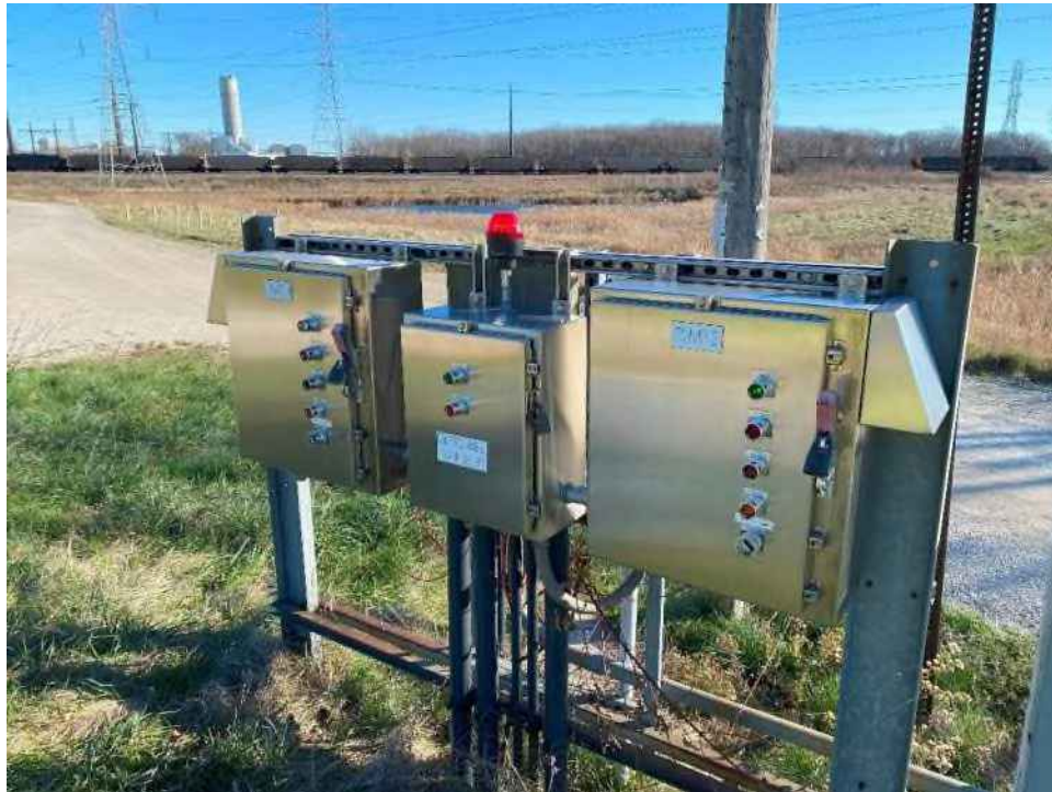
Photo No. 9 – Leachate tank control panel.
