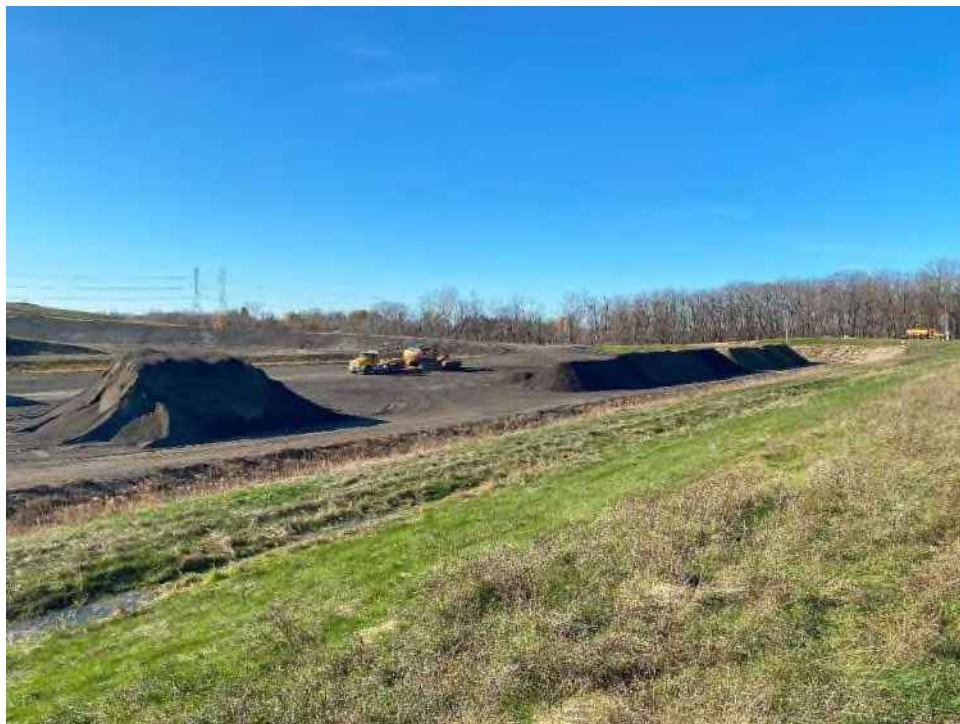
Photo No. 8 – Cell 10 active area. Contractor notified that piles need to be graded and compacted.
