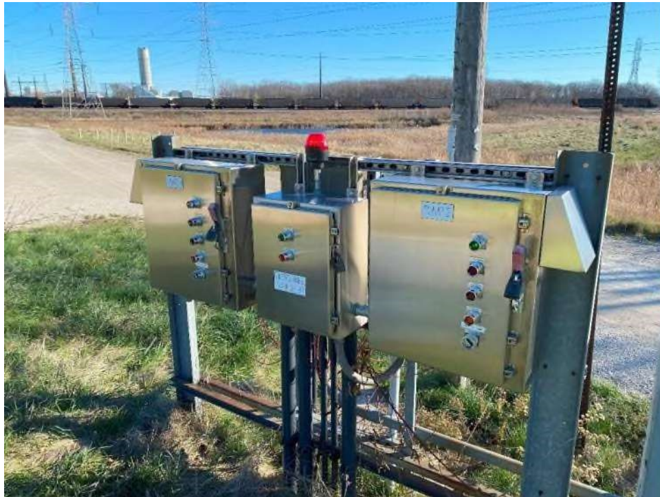
Photo No. 9 – Leachate tank control panel.
