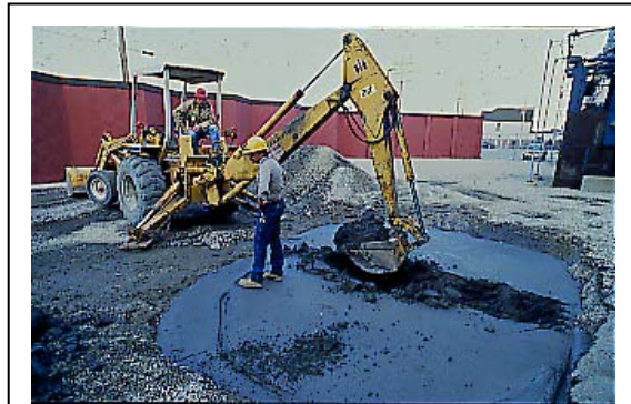
Figure 5-9: Excavating hardened CLSM with a backhoe at We Energies' Valley Power Plant in downtown Milwaukee, Wisconsin.
