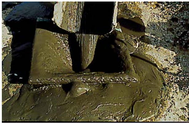
Figure 5-13: CLSM flowing through a funnel to fill an underground tunnel in downtown Milwaukee, Wisconsin.
