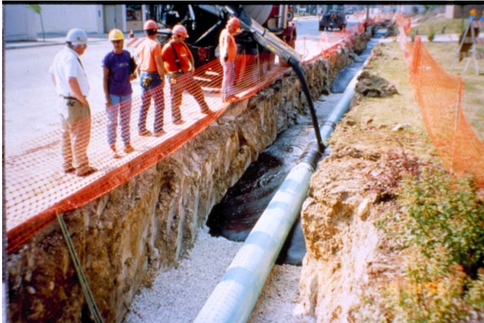
Figure 5-14: We Energies' Flo-Pac CLSM being placed in a direct buried steam pipe trench in downtown Milwaukee, Wisconsin.
